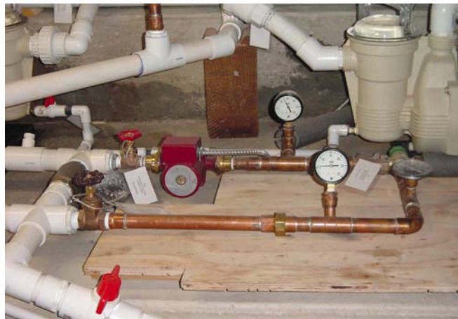
Detail of the pool loop.
