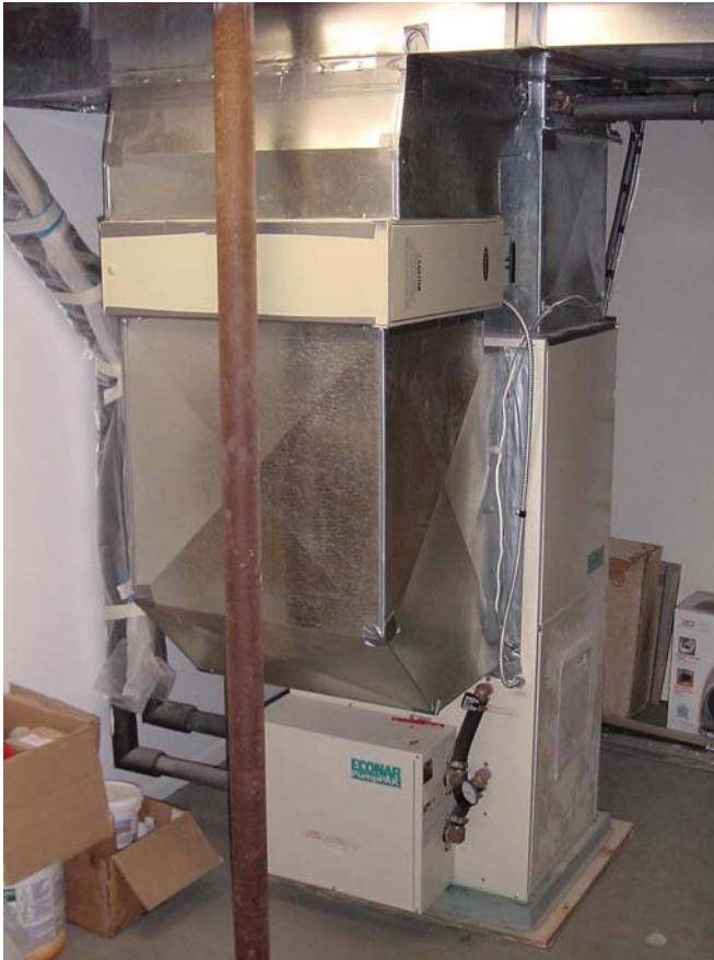
The Econar GeoSource heat pump adds to the system with heat from 3,000 feet of buried tubing.
