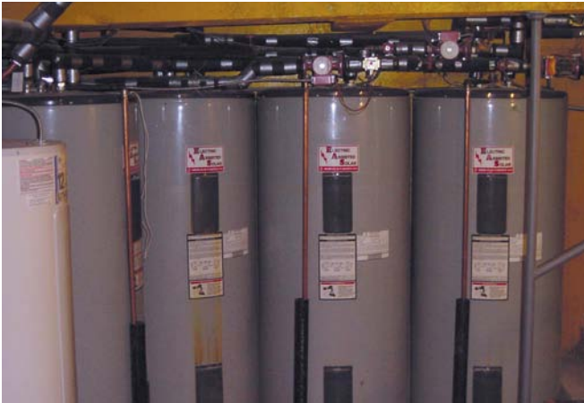
The water heater and four solar storage tanks.
